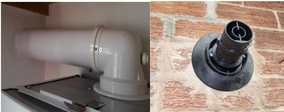
Figure 1 shows examples of correctly Secured and Sealed chimneys.
