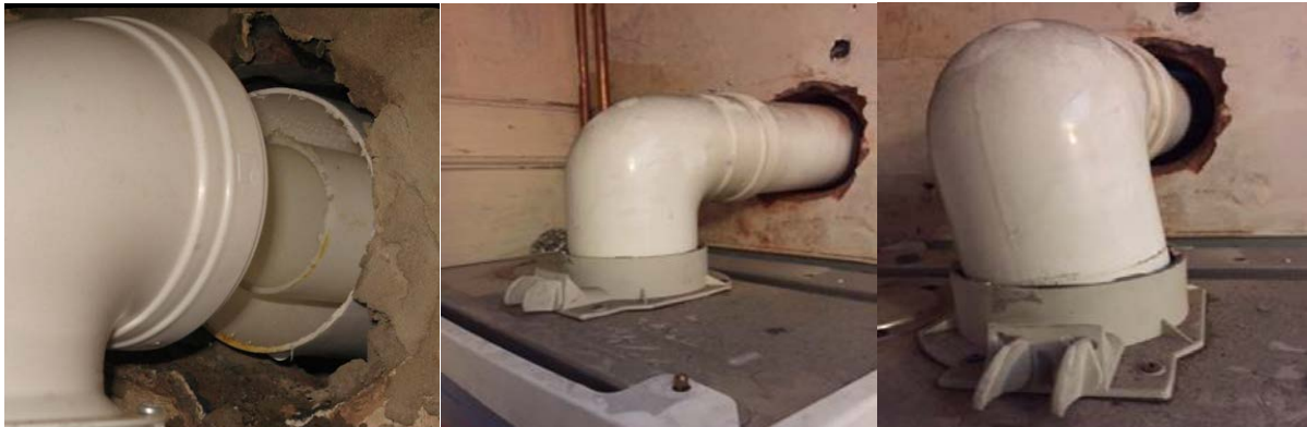
Figure 2 shows examples of incorrectly Secured and Sealed chimneys.
