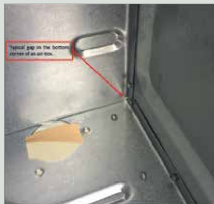
Typical gaps in air-box
